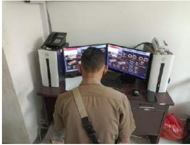
Sistem CPA ( Central Plan Automation ) chiller Gedung IMERI
